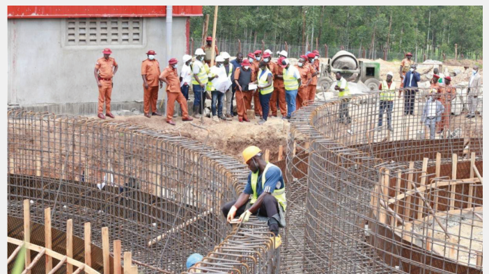
The CGP and senior officers from Prison Headquarters during an inspection of the ongoing site construction at Ruimi Prison Farm
